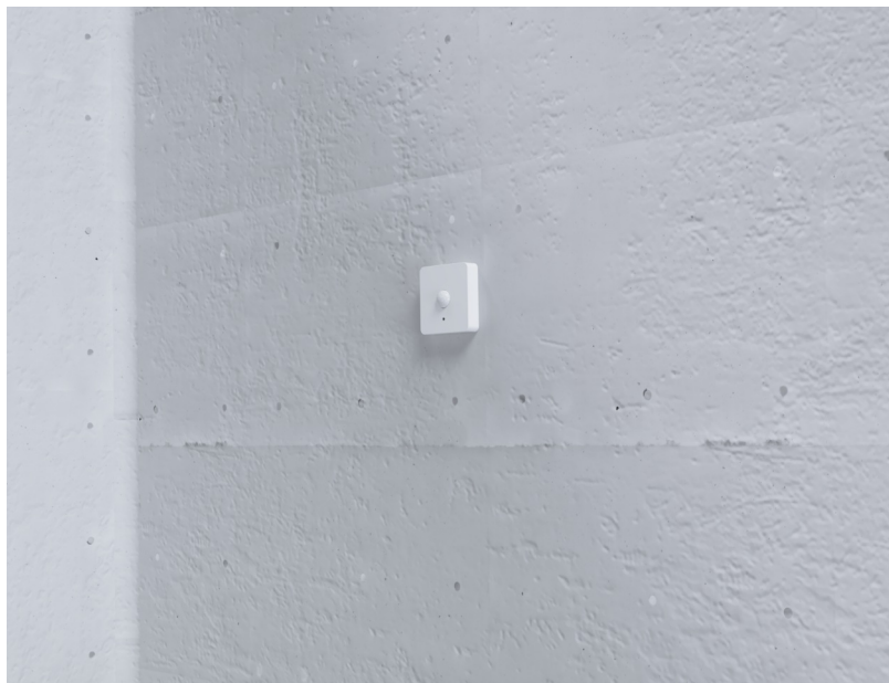
Fig 6: Wall Mounted presence sensor
