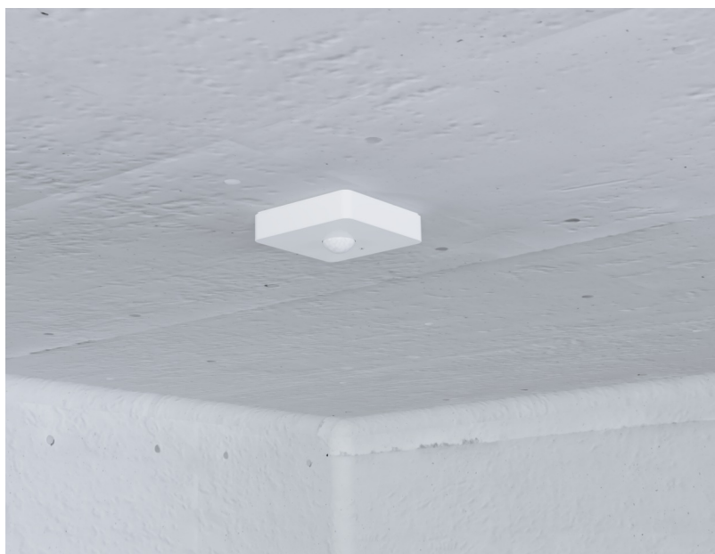
Fig 5: Ceiling Mounted presence sensor
